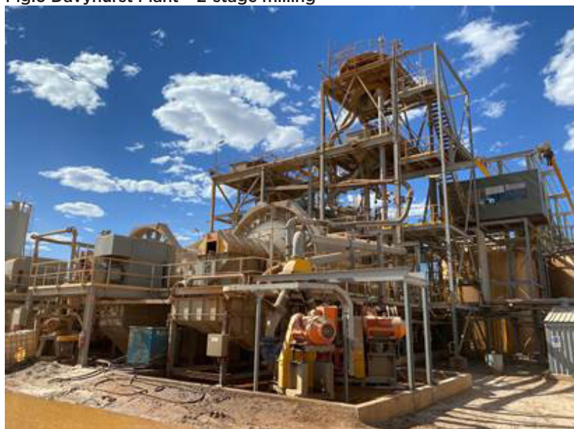
Fig.6 Davyhurst Plant – 2-stage milling
